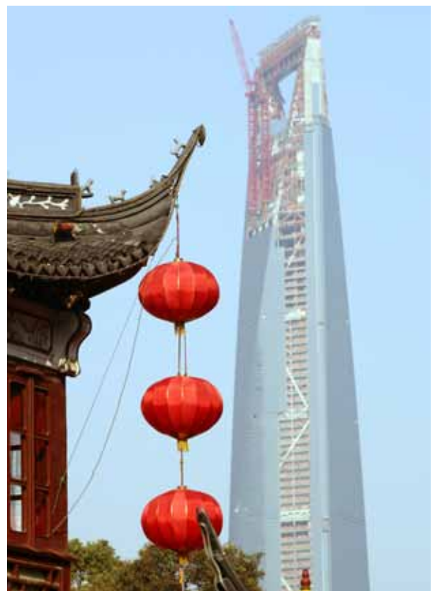
World Financial Center in construction, Shanghai, China (2008). The design, using a diagonal-braced frame, employs an effective use of material, because it decreases the thickness of the outer core shear walls and the weight of the structural steel in the perimeter walls
