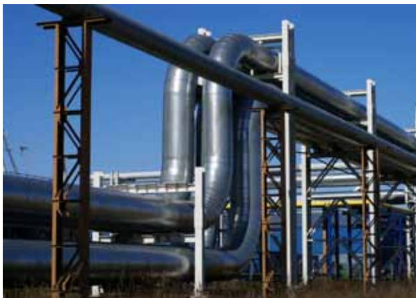
Industrial steel pipelines
